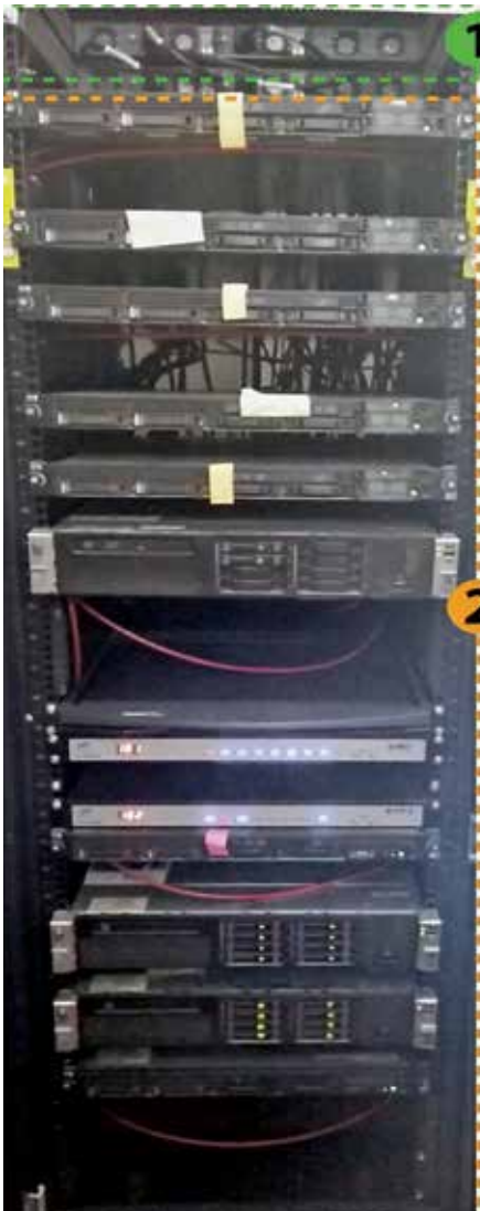
1. Fiber Channel Switches (2 Nos Active – Passive Mode)
